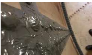
Steel tank rivet leaks – 251
