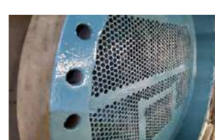
Heat exchanger/chiller – 200HT
