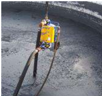
Corrosive sludge transfer
