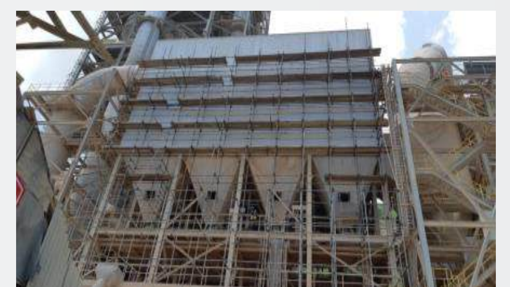
Flue gas – 200HT
