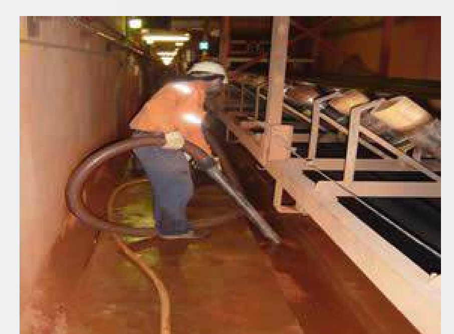
Accumulated mud and hard solids were removed from this canal with a Supavac pump.
