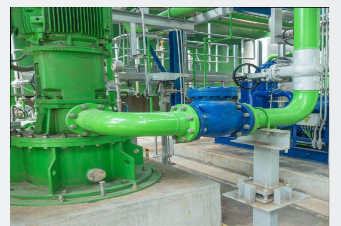
Plant wide corrosion and abrasion protection
