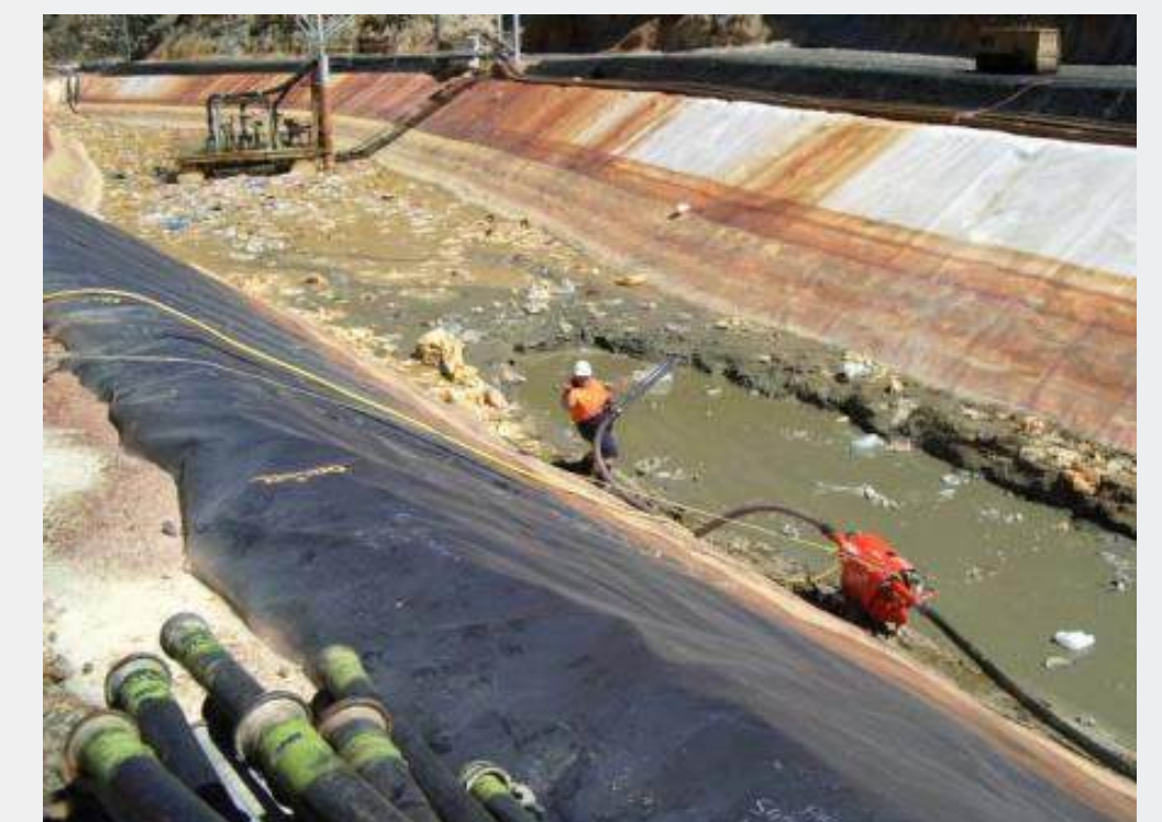
Accumulated mud and hard solids were removed from this canal with a Supavac pump.
