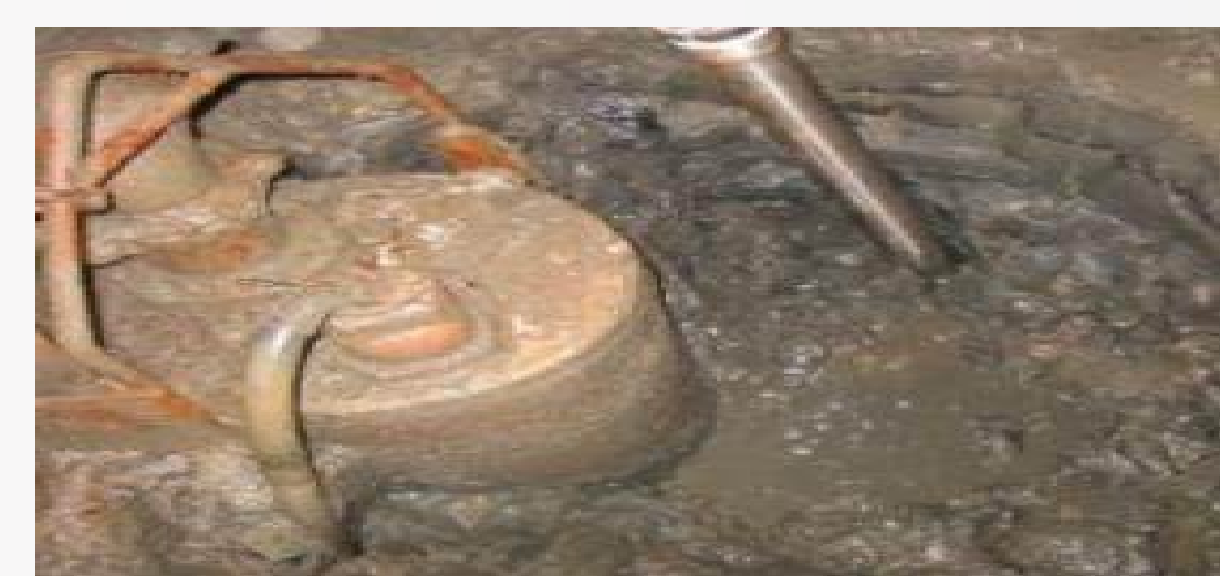
This overwhelmed submersible pump rescued, repaired and returned to service.
